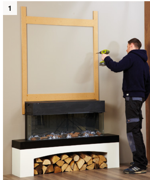
The support frame is fixed to the wall leaving a small gap above the fire to avoid resonance.
